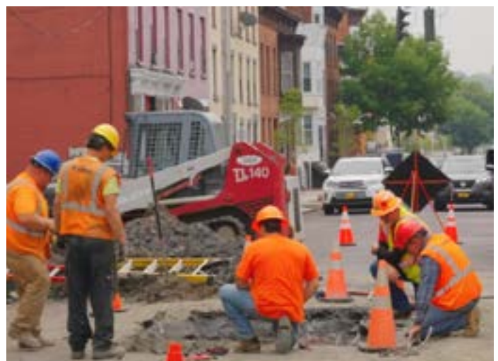
Lead pipes being replaced as part of Troy's Lead Service Line Replacement Program. Image from troyny.gov.
